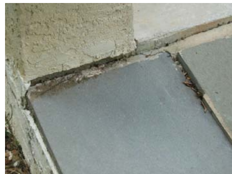
Settled Patio Flagstone (typical)
