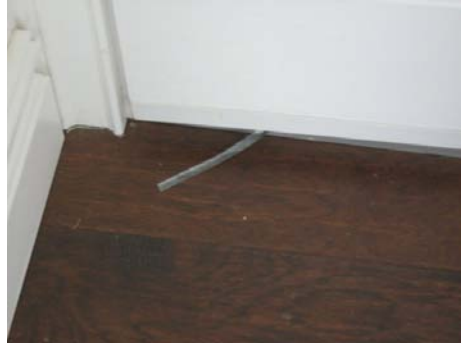
Damaged Weather Stripping
