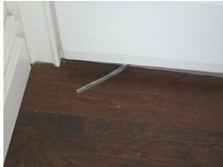
Damaged Weather Stripping
