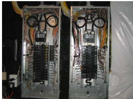
Electric Distribution Panels
