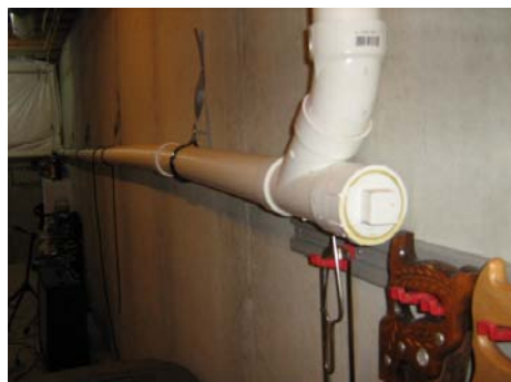
Improperly Sloping Waste Piping
